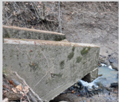
Erosion at outlet
