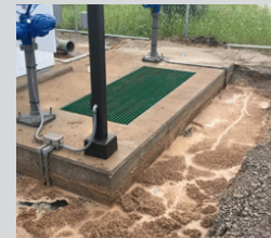
Collector system is compromised
